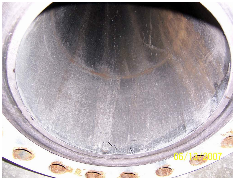
Figure 17: 12-inch Dirty Piping
