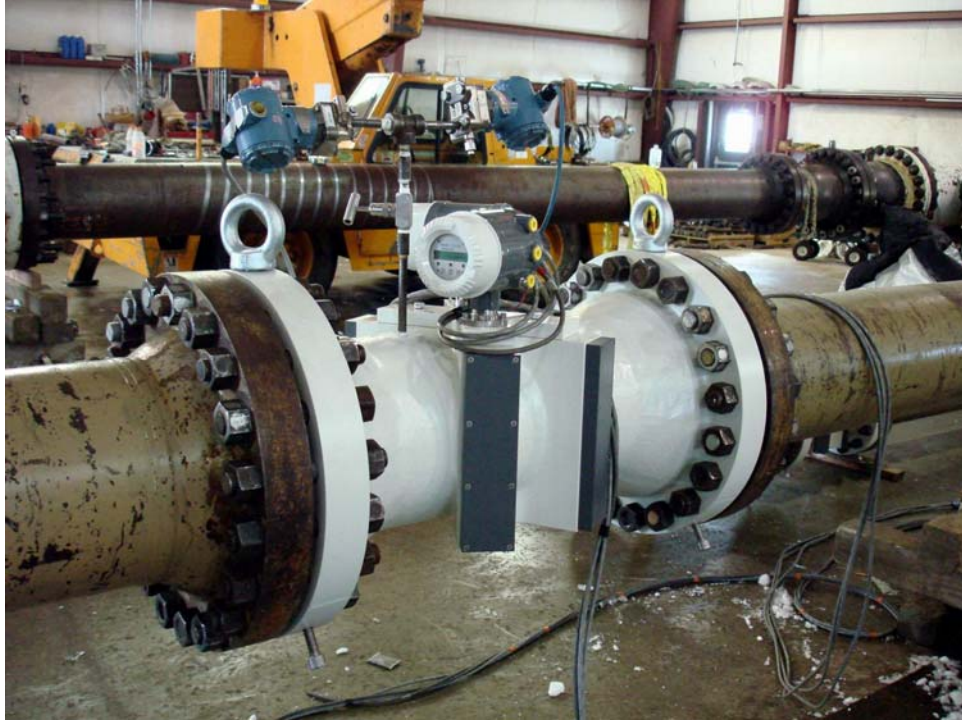
Figure 5: 12-inch 4+1 CBM Meter CEESI
