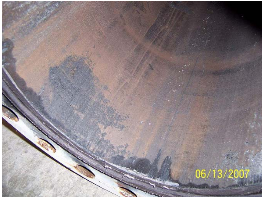
Figure 18: 12-inch Dirty Piping Close Up
