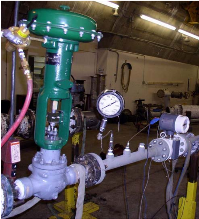
Figure 8 – Control Valve near 2-inch USM
