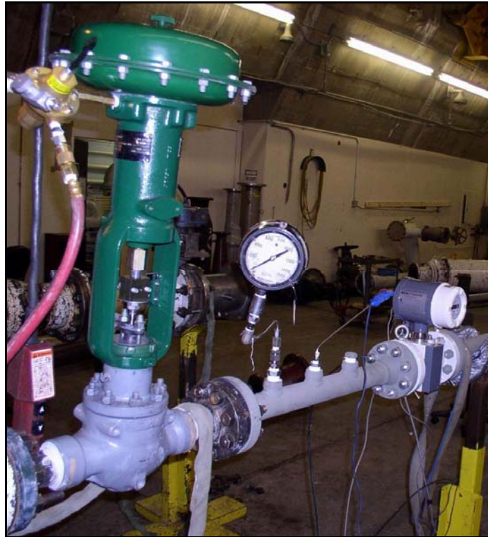
Figure 14 – Control Valve Piping
