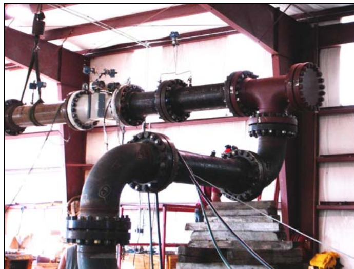
Figure 40: 8-Path Meter with PTB Flow Conditioner Piping
