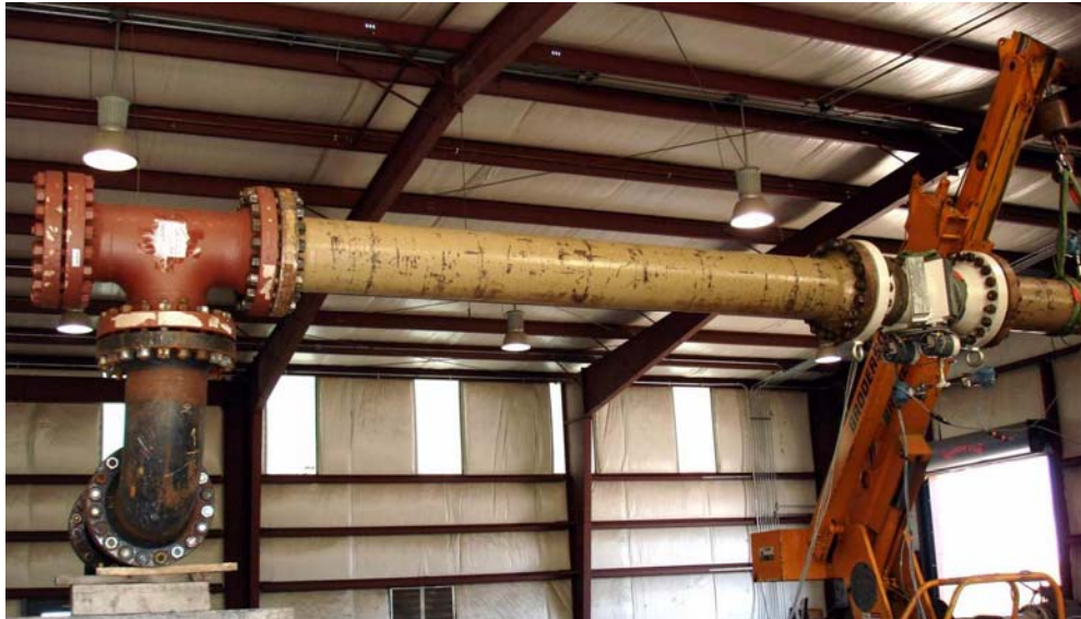
Figure 26: 8-path Meter at 10D No Flow Conditioner
