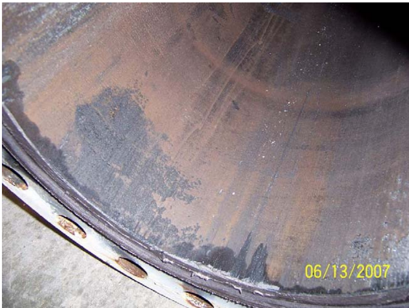
Figure 18: 12-inch Dirty Piping Close Up
