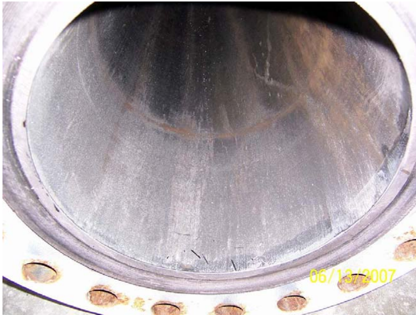
Figure 17: 12-inch Dirty Piping
